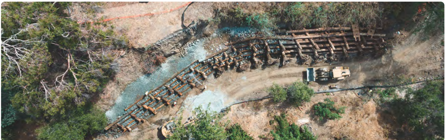
Construction of the crib wall for the Children's Health Council School, San Francisquito Creek Bank Stabilization project.
