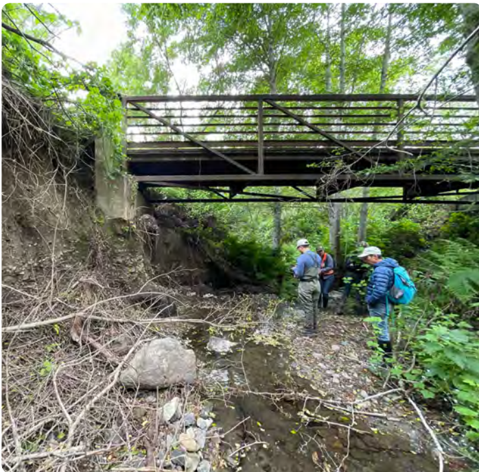
WRA inspecting bank erosion on the Middle Fork of San Pedro Creek in a team effort with Consor to support San Mateo County Department of Public Works.
