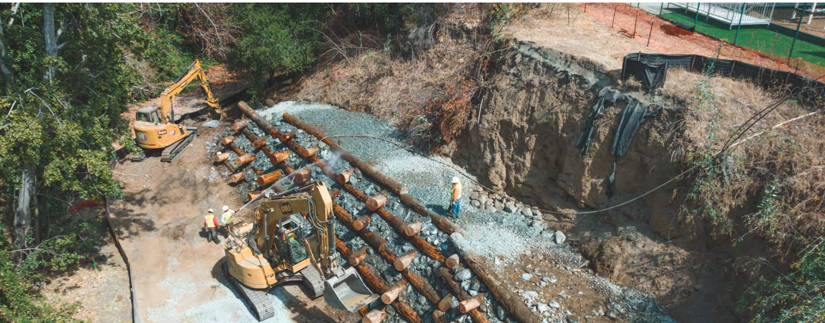
Construction Crews installing gravel filter layer over crib wall prior to placing native soil and riparian plantings for the Children's Health Council San Francisquito Creek Bank Restoration project.
