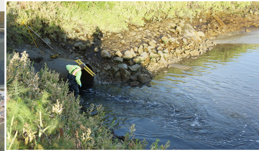
New wastewater effluent outfall
