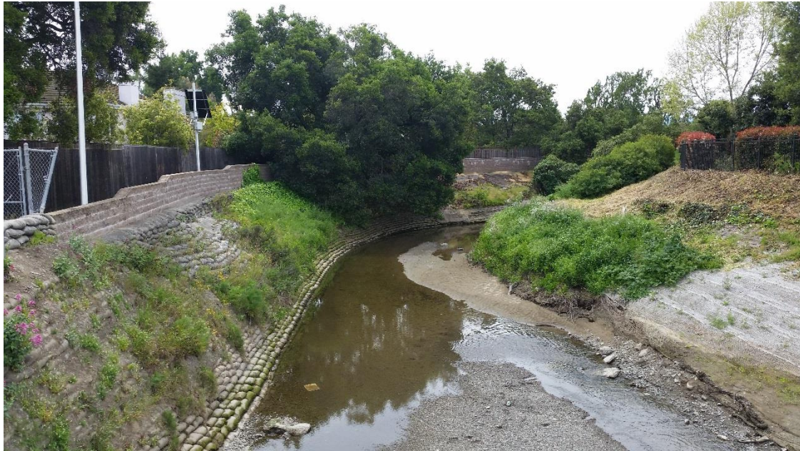
Overview of San Francisquito Creek, directly south of the University Avenue Bridge, view south
