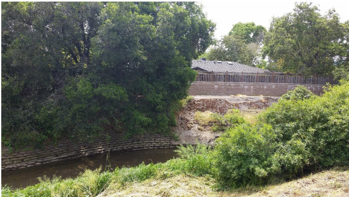
Overview of San Francisquito Creek, directly south of the University Avenue Bridge, view southeast
